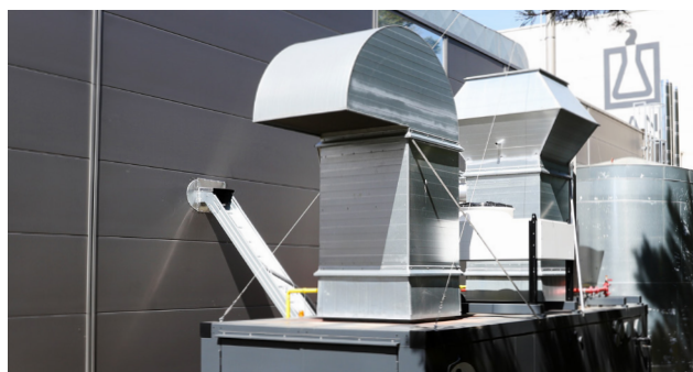
CHP station at BRAND KG
